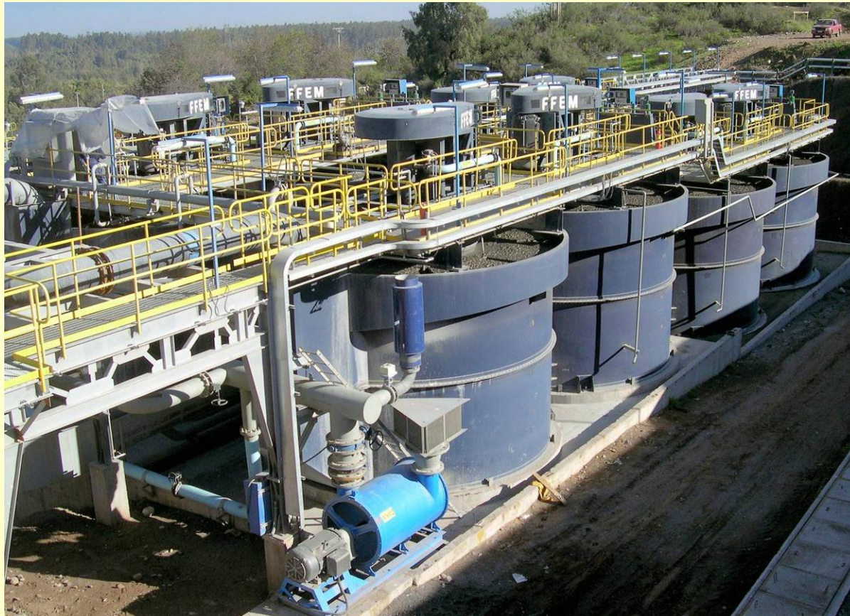
View of the 16 x 160 m 3 FFEM Cells Installation
